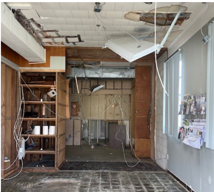
The SVCA and Trust offices took most of the water damage. Our work party of extraordinary volunteers had it gutted in no time!
